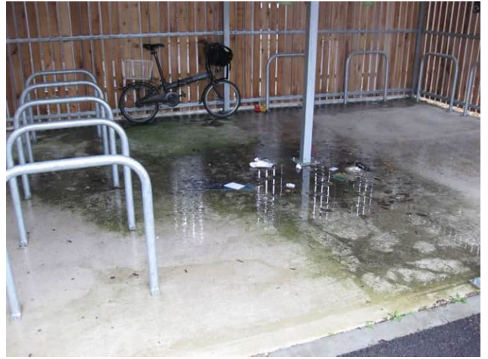
Figure 33: covered parking in Parker's Trade Park in Bedford Road showing a puddle and patches of slippery green slime, together with litter.
