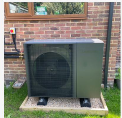
Enabling works for an Air Source Heat Pump installation supported by subsidised capital grant funding.
