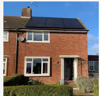
Solar PV installation supported by subsidised capital grant funding.
